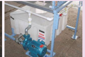
150 litres disinfectant solution tank
